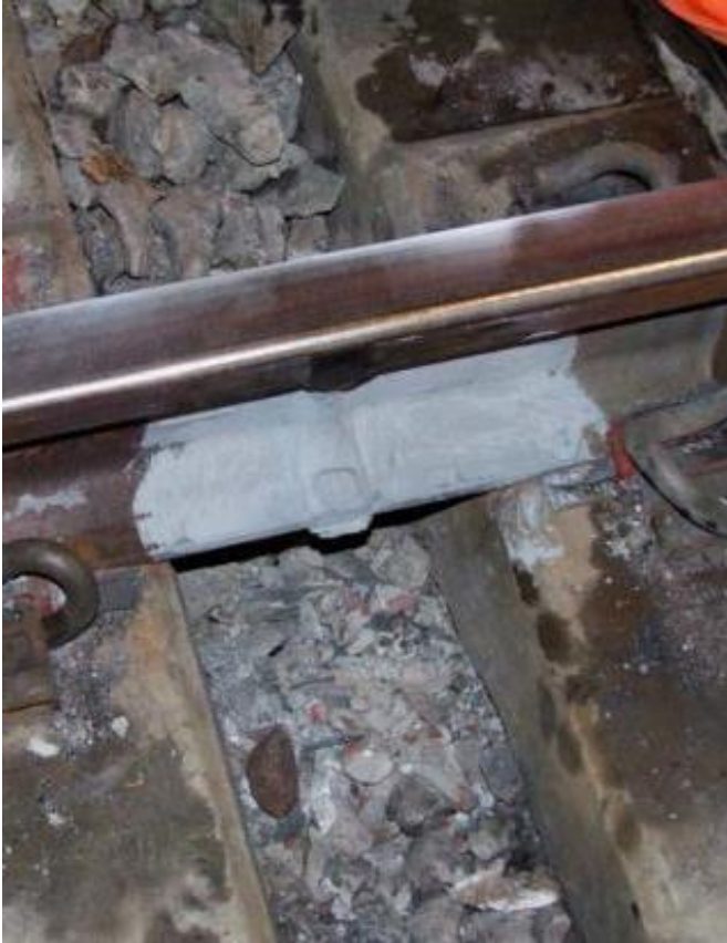
Example of the “touch up” procedure applied to an aluminothermic weld. N.B. Image is of an uncoated rail to highlight “touch-up” area.
